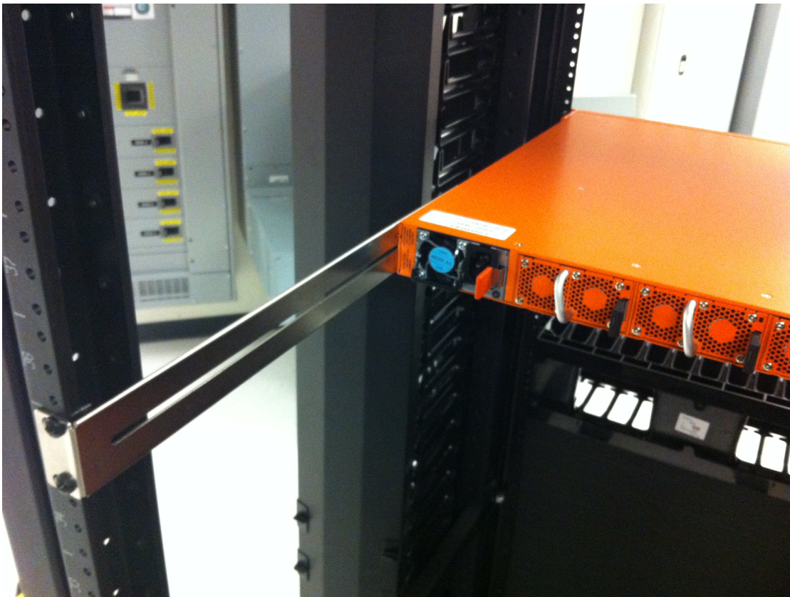
Figure 4 Rear View of the Mounted Node and Rails on the Four-Post Rack
